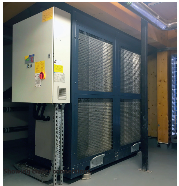
Below: The HFO chiller in situ in the plant room.
